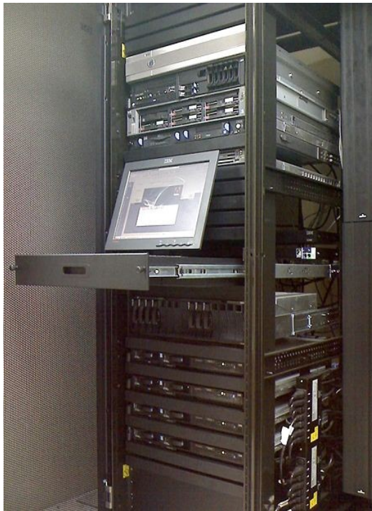
Front of a rack
